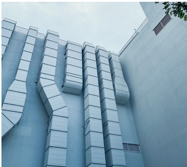
Figure 5. Melamine duct insulation systems.
